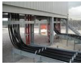
CABLE TRAY PROTECTION
