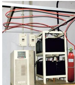
UPS PROTECTION at Agni Controls, Chennai (Unit-3, Vyasarpadi)
