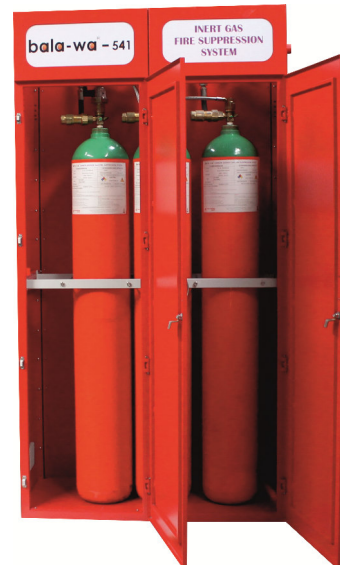
balawa-100/541 Inert gas suppression system using Master and Slave Operation
