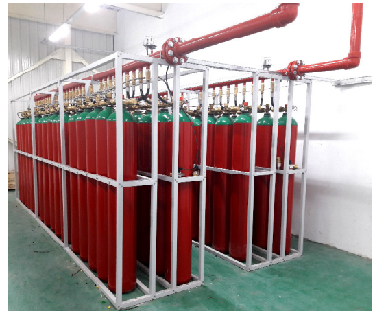
balawa-100/541 inert gas suppression system using Master and Slave Operation
